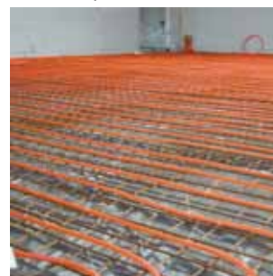
Industrial floor heating
