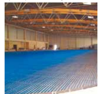
Chilled area, ice stadium
